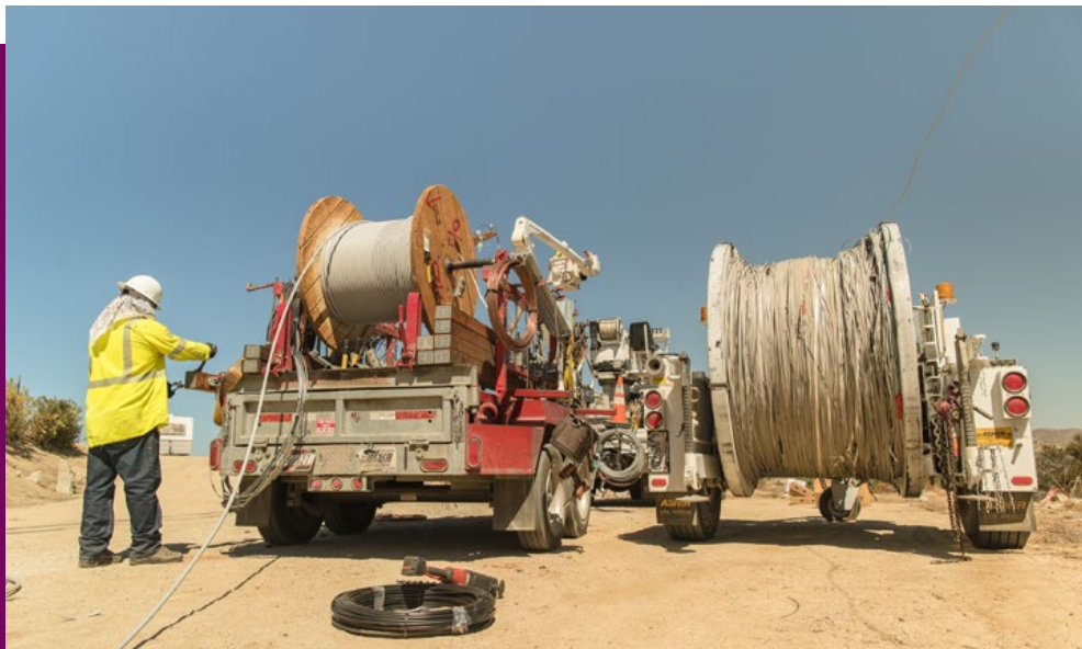
Covered conductor, a key tool in our wildfire mitigation efforts, is insulated wire that eliminates the risk of ignition when debris blows into lines during high winds.
