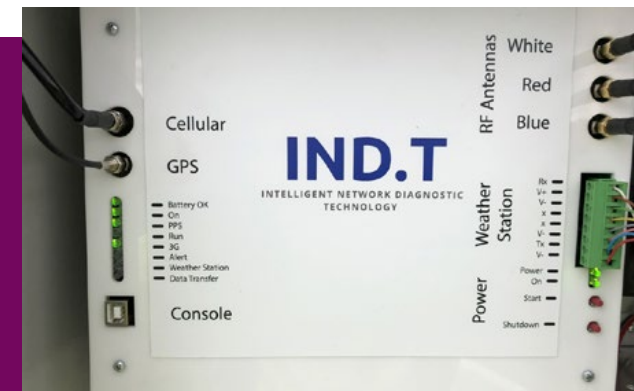
SCE is piloting Early Fault Detection technology — devices that are installed on power poles and listen in on the electrical noise coursing through power lines — to help detect and mitigate against disruptions related to electrical infrastructure that could lead to wildfire hazards.
