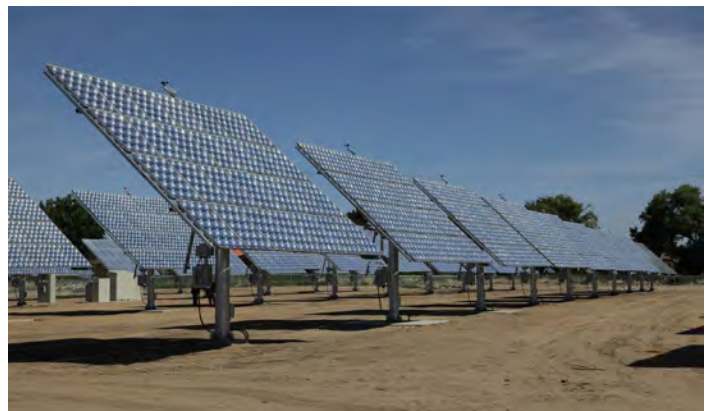
Solar panels at Victorville Community College.
