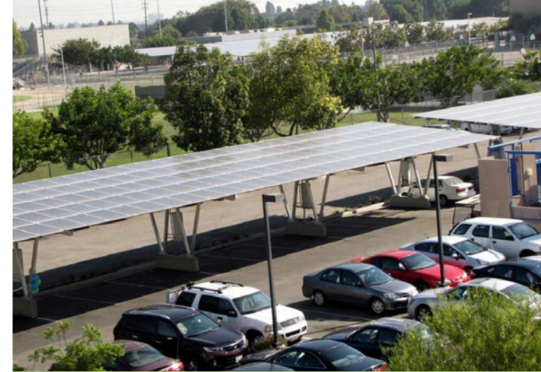
SCE-supported solar carport project in Long Beach
