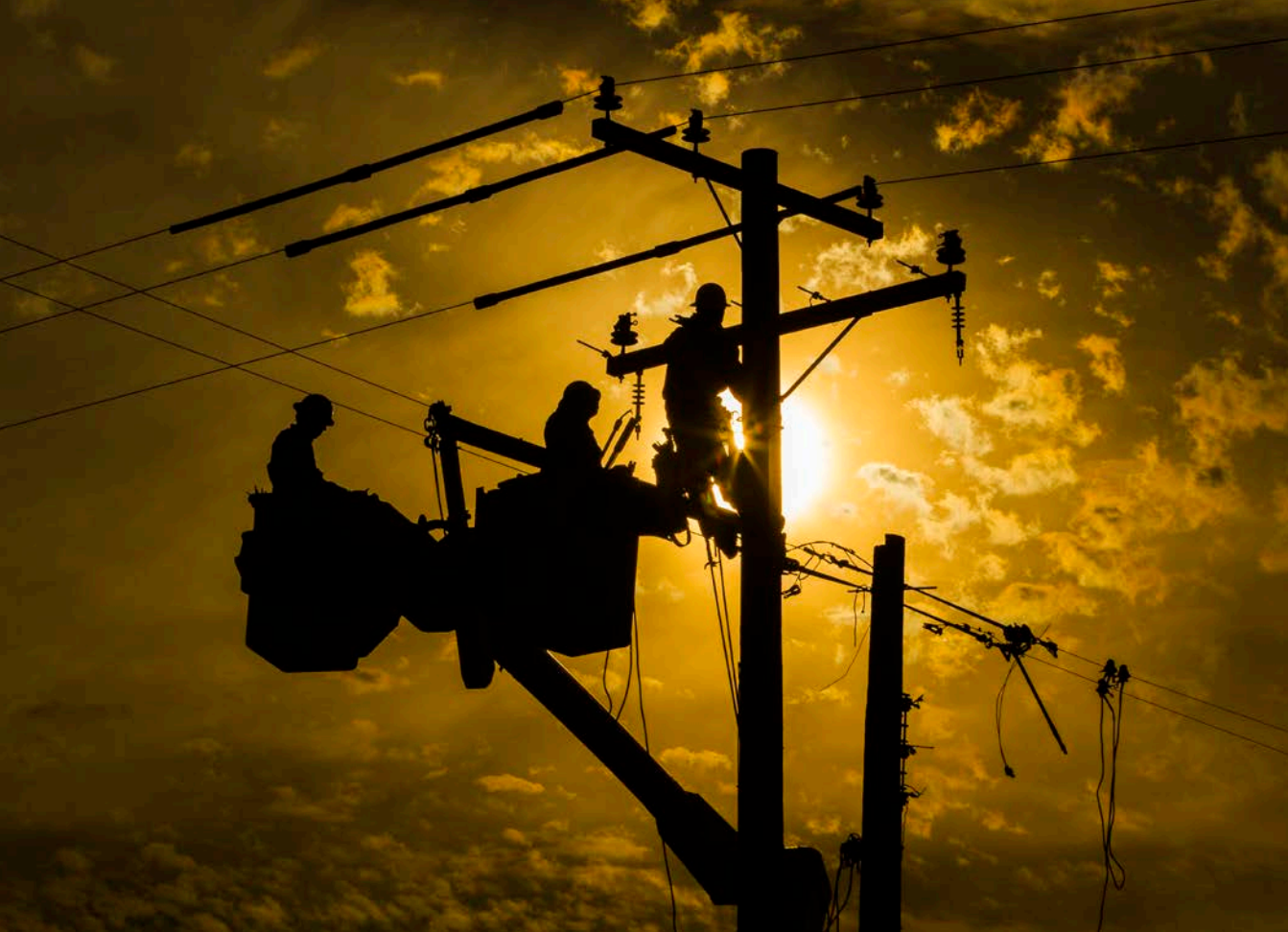
Linemen attend to one of SCE's nearly 1.5 million utility poles.
