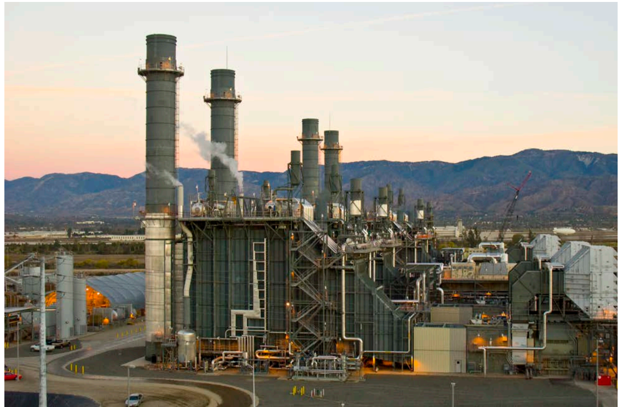
SCE's Mountainview power plant recovers and recycles 80 percent of the water used in its cooling process.
